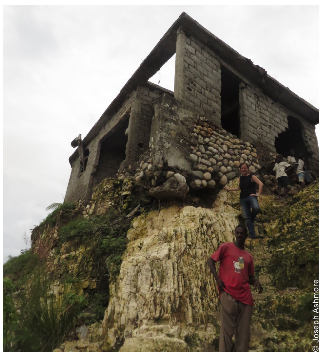
Houses in informal settlements are often vulnerable due to poor locations (marginal sites), poor materials (here we have river stones for foundations) and poor construction.
