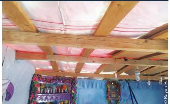
Before installation of the insulation kits, poor quality plastic sheeting and other temporary materials, such as cardboard, were commonly used in most of the shelters targeted by this project.
