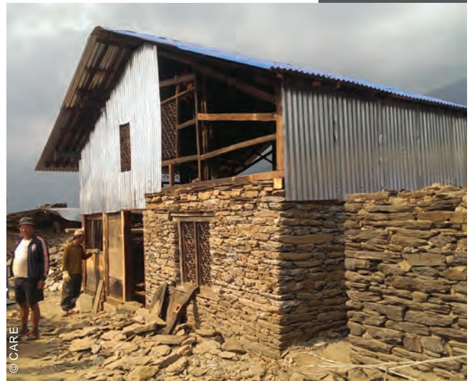
In response to the Nepal earthquakes in 2015, humanitarian organizations adopted a variety of response modalities, including distribution of CGI sheeting to repair damaged structures, particularly to prepare for the harsh winter season.
