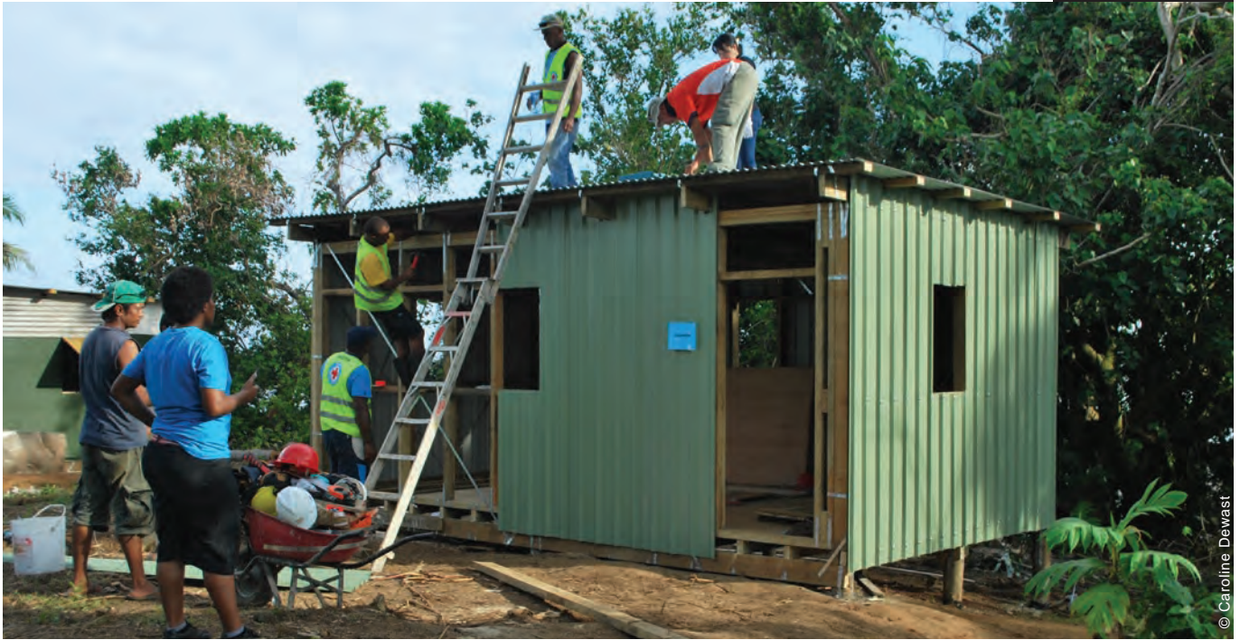
Build Back Safer trainings were the key component of the Shelter Cluster strategy.
