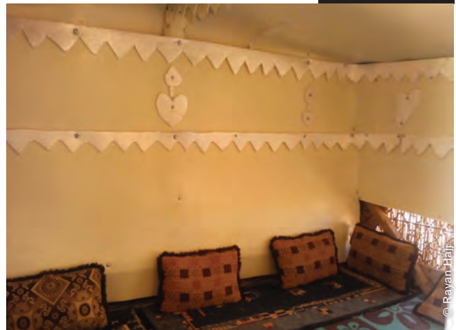
The insulation foam was to be applied to both walls and ceilings, and in some cases people were creative and made decorations out of the same material.
