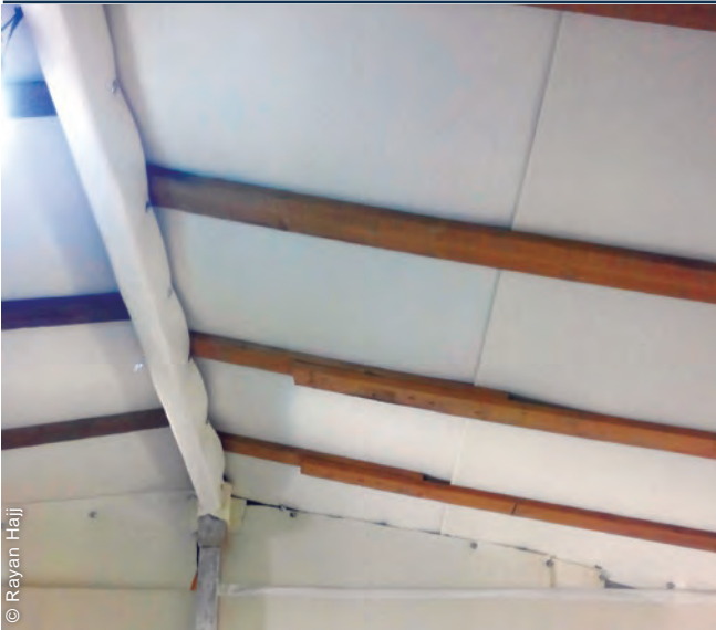
People installed the insulation foam to reduce the heat loss, which generally tends to be higher through the ceiling/roof and the floor/ground.
