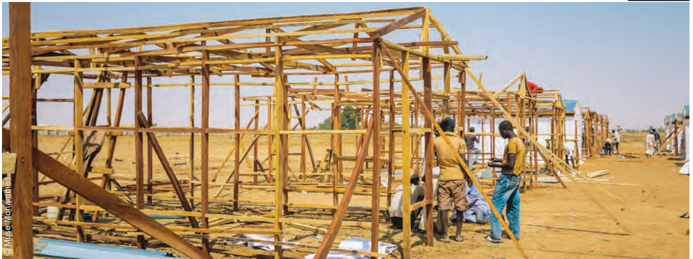
The shelters were built by contractors, with the condition that they hired workers locally including IDPs, who received on-the-job training.
