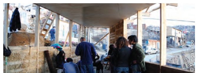
Local groups of architects organized building workshops to rebuild some of the houses affected by the fire on the Quebradas.
