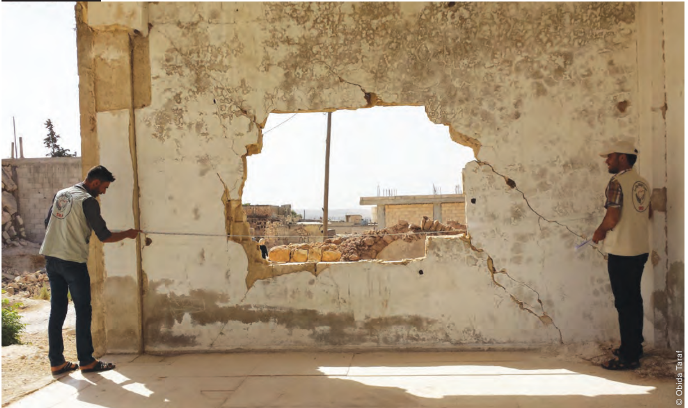
Given the very different operating environments, different responses took place in different countries. To promote some consistency, the Whole of Syria approach was adopted in 2013. In this picture we see assessment for a housing repair project within Syria.
