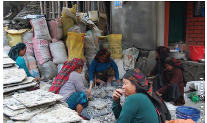
After the rapid gender analysis, the project consulted the communities, engaged women in construction activities, and aimed to meet specific gender needs in both distributions and construction (here, on a building site in Barpak).
