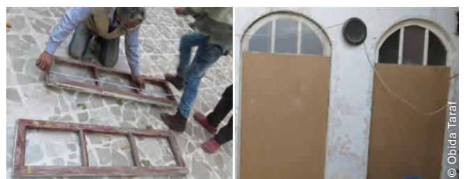
Repairs included the replacement of window frames or sealing off of openings.
