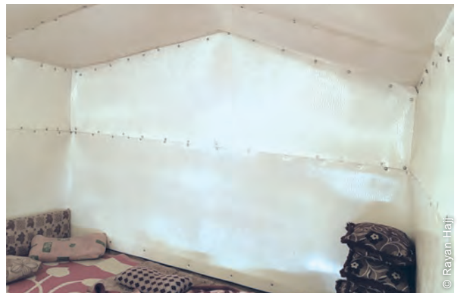
The foam was applied to walls and ceiling, while mats and pillows were used to insulate the floor. This achieved a full insulation of the shelter, which ensured a significant reduction of the heat loss during the winter, as well as good performance during the summer.
