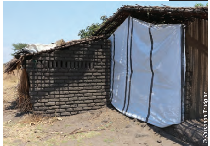
Tarpaulins from the shelter kits were used, amongst other purposes, to seal off damaged parts of the houses.
