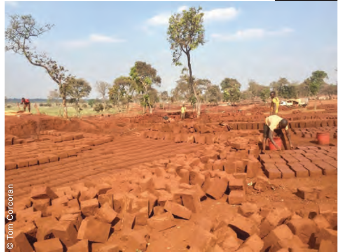
The process of adobe brick making in Nyarugusu refugee camp managed to produce a total of over 11 million bricks, used for the construction of the shelters.
