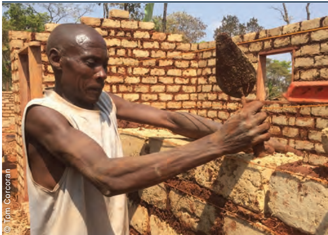
Mason laying the bricks of a shelter in Nduta refugee camp. Skilled builders from the refugee population were employed for the construction of the shelters.
