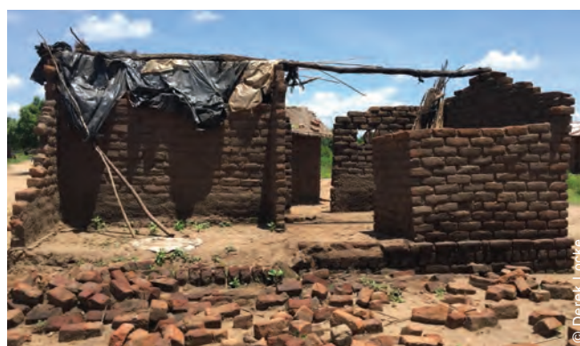
Some structures sustained significant damage due to the floods.
