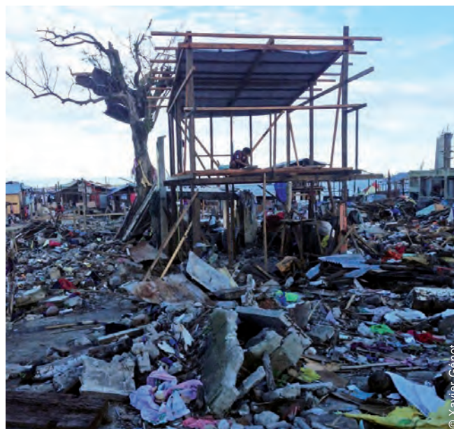
Many people rapidly started to build shelters after Typhoon Haiyan (here in Tacloban, December 2013).
