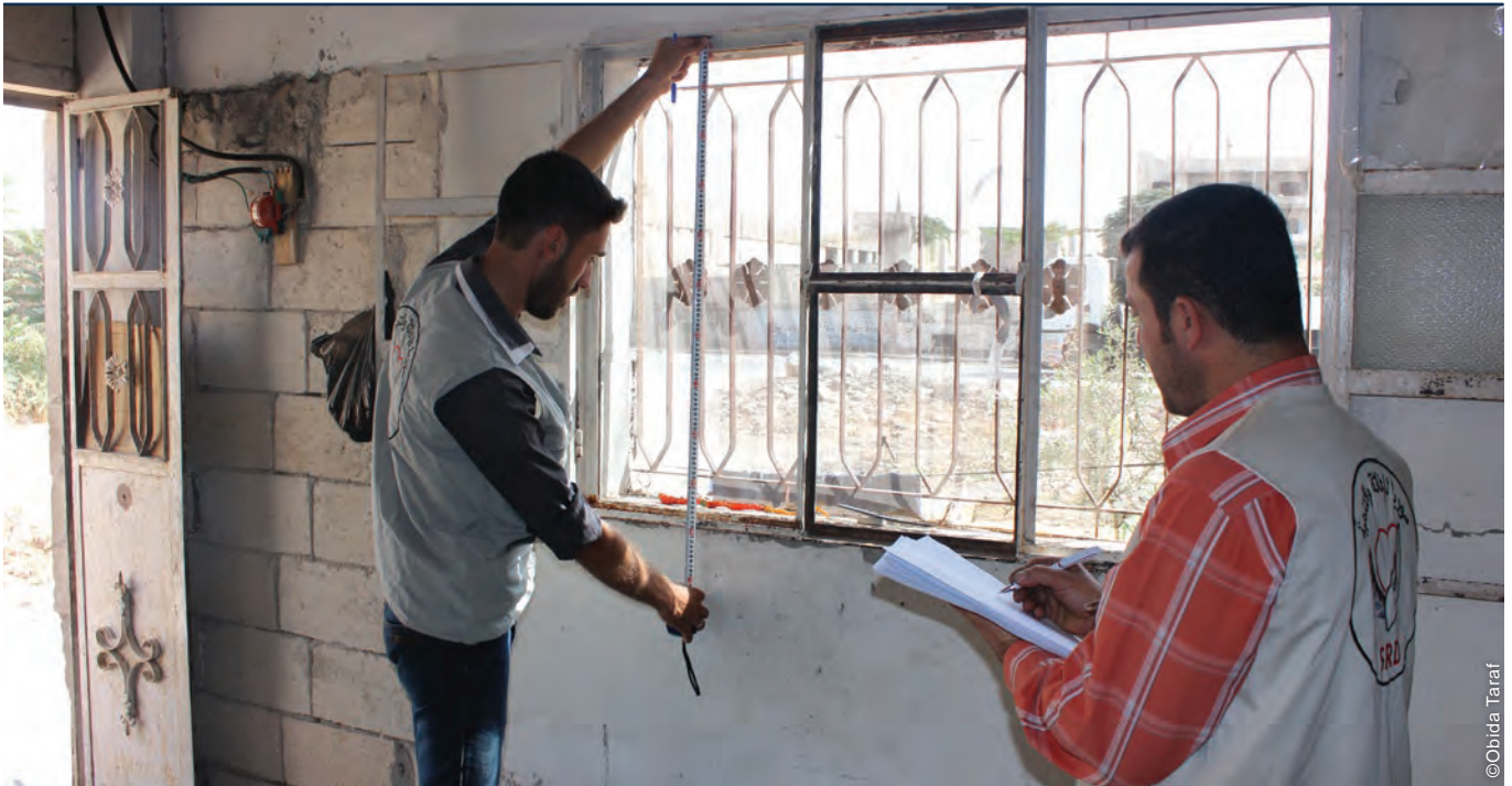
The project included repairs and upgrades to walls, floors, ceilings, doors and windows and installation of wiring, plumbing and latrines.
