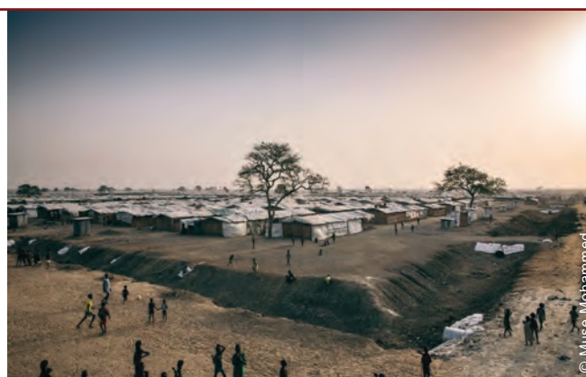
The site works were based on a Dutch "polder" system. They included 28m 2 section drainage ditches, berms, water retention basins, and large volume pumps to evacuate water.
